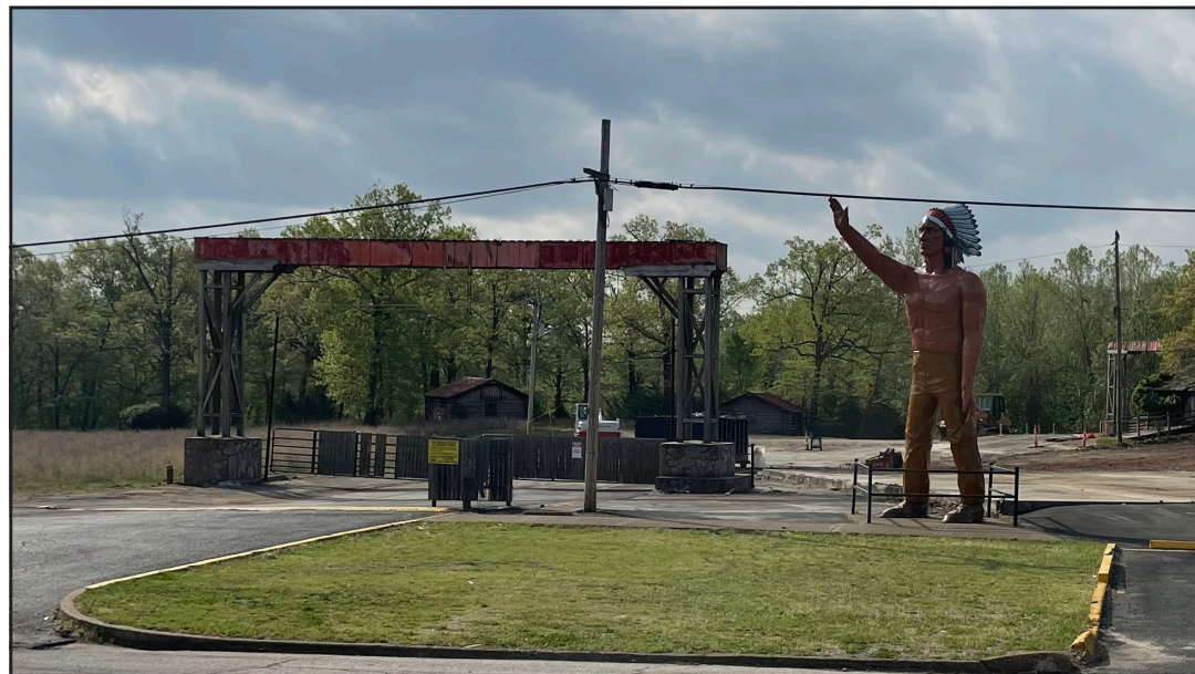
Reese Development recently completed demolition work along the historic Bagnell Dam Strip in the City of Lake Ozark to make way for new development
